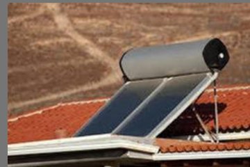
Solar Power Installation
