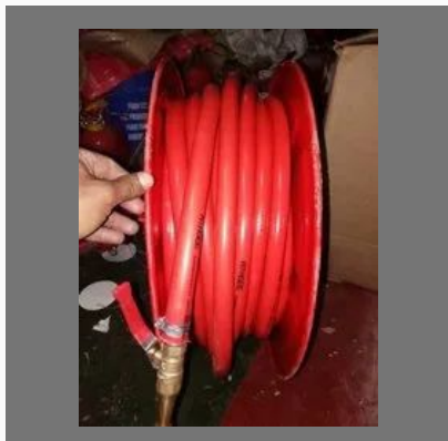
Fire Hose Reels
