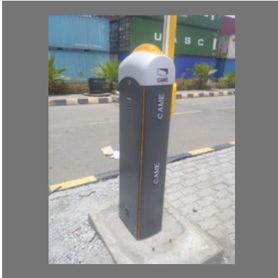
Boom Barrier - Port Gate Automation
