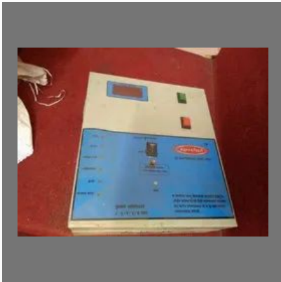
Motor Panel Box
