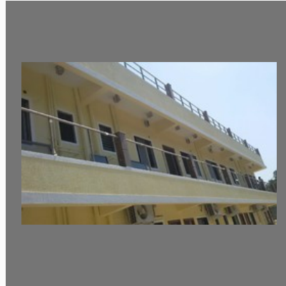
SS Balcony Glass Railing
