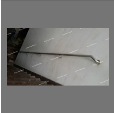
Stainless Steel Handrailing
