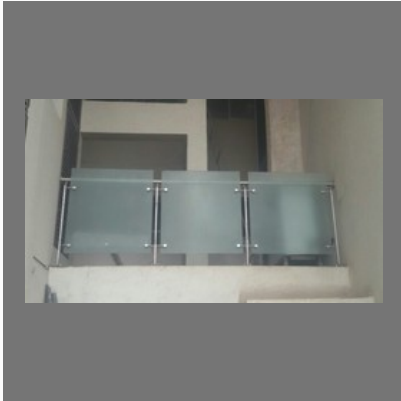
SS Balcony Glass Railing
