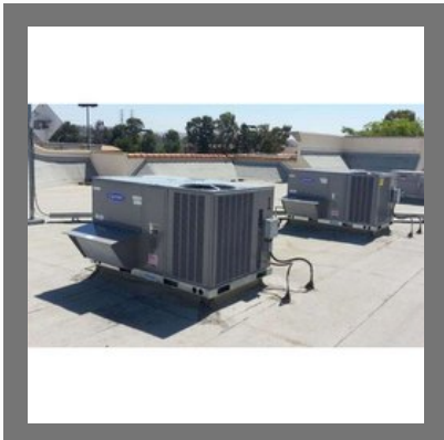
Automatic HVAC Units
