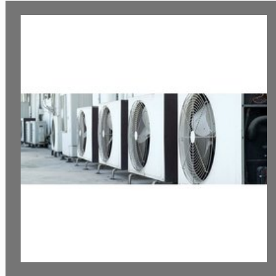
Automatic VRF Systems
