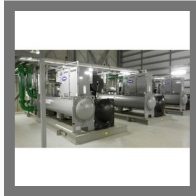
Air Conditioning Plant
