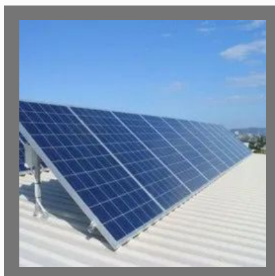
Rooftop Solar Power Panel
