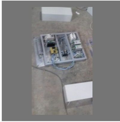
Electric Control Panel
