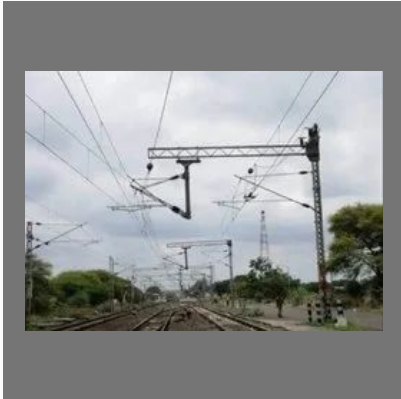
Railway OHE Mast
