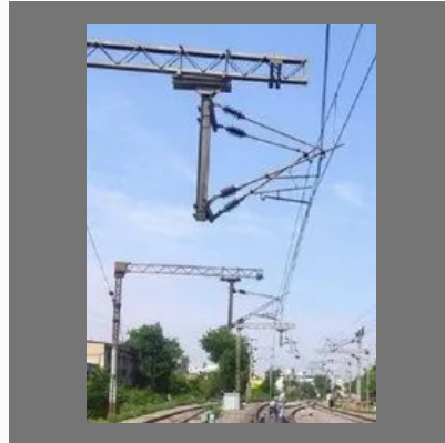
Railway TTC Mast Poles
