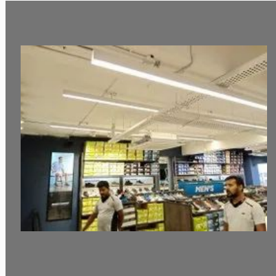
Lighting Wiring Services
