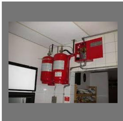
Kitchen Fire Suppression System
