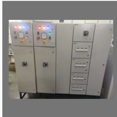
Electric Control Panel
