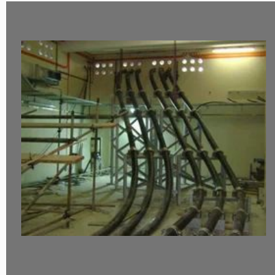
Electrical Turnkey Projects
