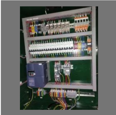
VFD Electrical Panel
