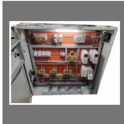
MCC Electrical Control Panel
