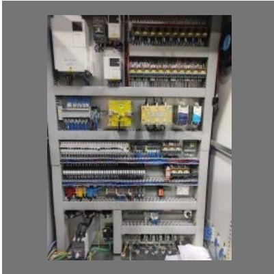
Motor Control Panel
