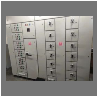
SS Electrical Distribution Control Panel
