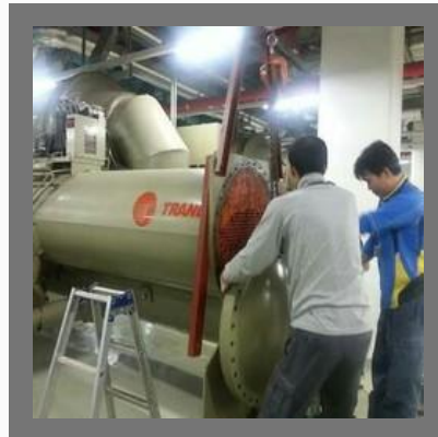
Chiller Plant Cleaning Services
