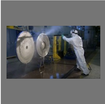
Condenser Cleaning Services
