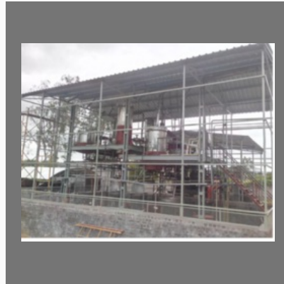
Jaggery Powder Plant
