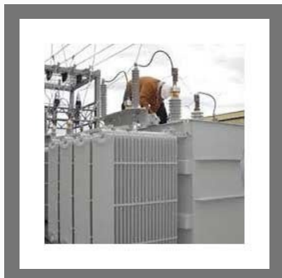
Substation AMC Service
