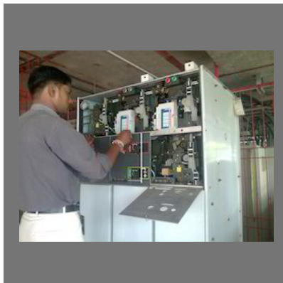
Circuit Breaker Maintenance Services
