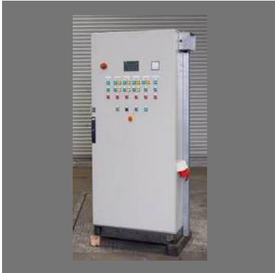
Belt Conveyor System Panels
