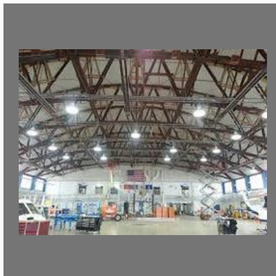
Industrial Lighting Service
