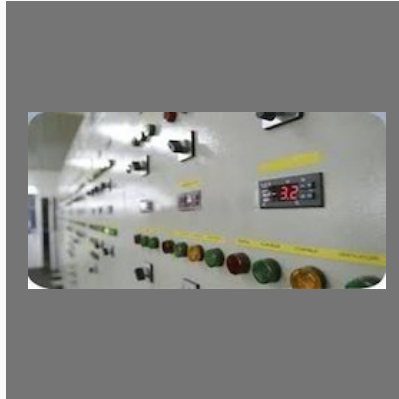
Control Panel For Food Processing Industries
