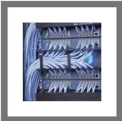
Structured Cabling Solutions
