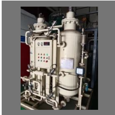
Industrial Compressed Air Dryer Services
