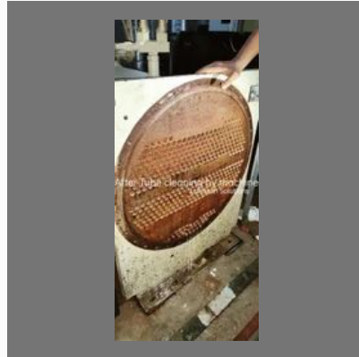
Chiller Descaling Service
