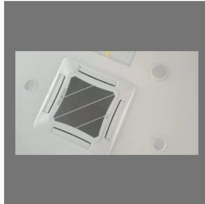
Cassette Air Conditioners Installations
