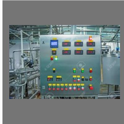
Dairy Plant Control Panel
