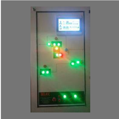
Electric Control Panel
