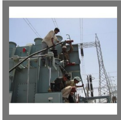
Transformer Maintenance Services
