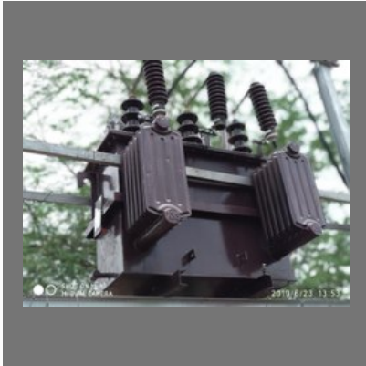
Three Phase Oil Cooled Power Transformer
