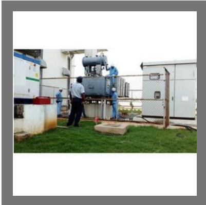
Electrical Transformer AMC Services
