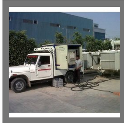
Transformer Oil Filter Services
