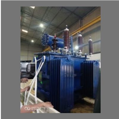
200 KVA Distribution Transformer
