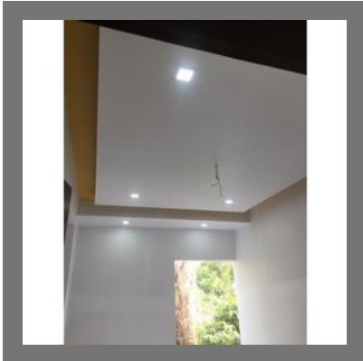
Sakrani POP False Ceiling
