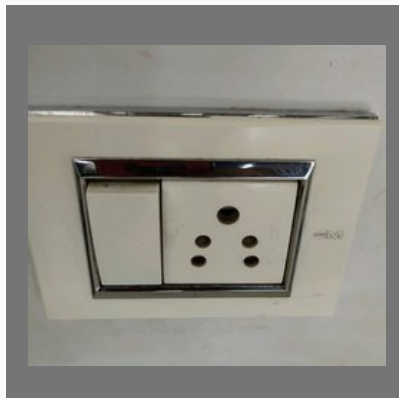
Home Electrical Switches
