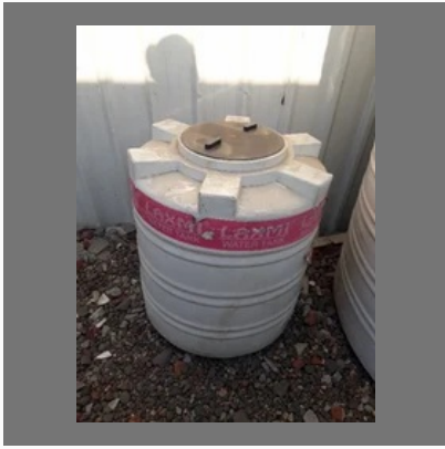
Water Storage Tanks
