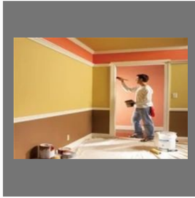
Plumbing And Interior Services
