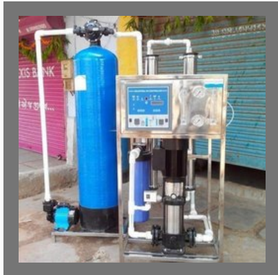
Automatic Stainless Steel Reverse Osmosis Plants
