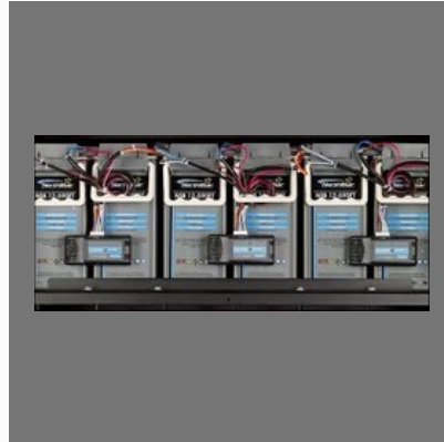
Battery Health Monitoring System
