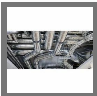
HVAC Air Duct
