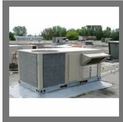
Commercial HVAC System
