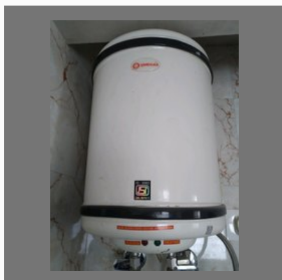
Electrical Water Heater
