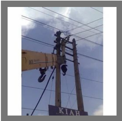
Industrial Electrical Contractor
