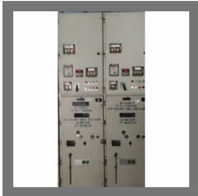
Vacuum Circuit Breaker
