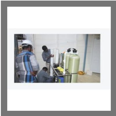
Industrial RO Plant Maintenance Service
