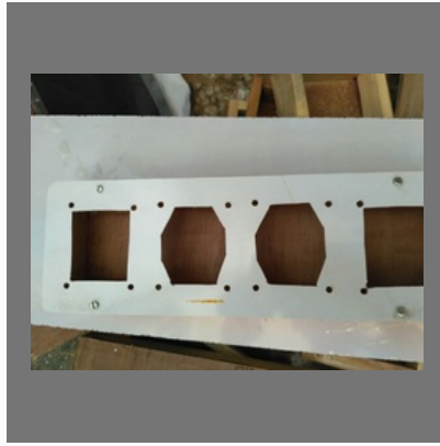
Electric switch board
