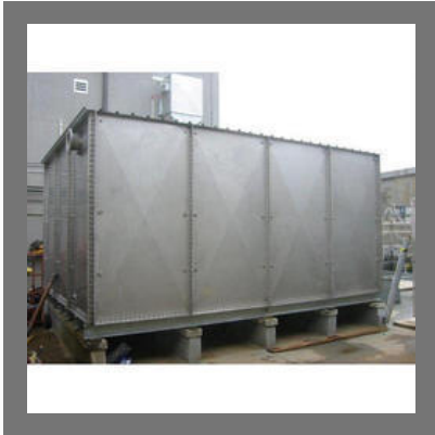
Mild Steel Storage Tank
