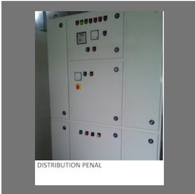
Distribution Panel Box
