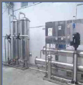
Commercial Water Treatment Plant
