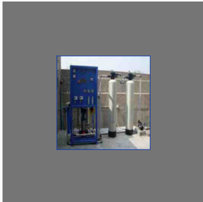
Domestic Water Treatment Plants
