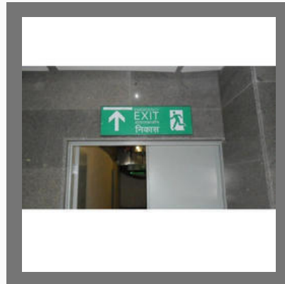
Exit Sign Board
