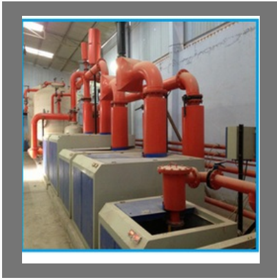
VPSA Oxygen Plant
