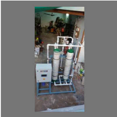
ULTRA FILTRATION PLANT
