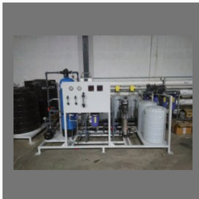
Commercial Reverse Osmosis Plant
