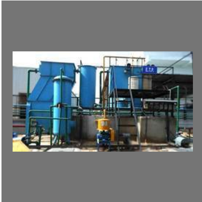
EFFLUENT WATER TREATMENT PLANT
