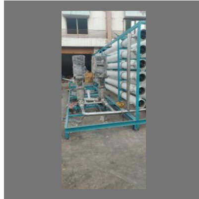
INDUSTRIAL WATER TREATMENT PLANT
