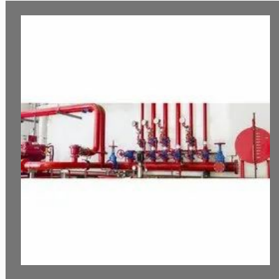
Fire Protection Systems
