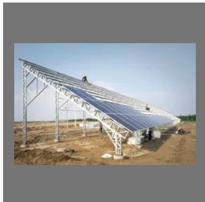
Solar Panel Mounting Structure
