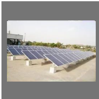
Solar Panel Rooftop Mounting Structure
