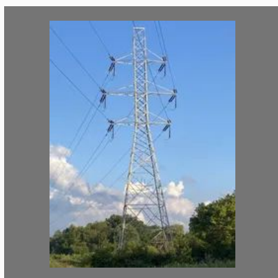
Mild Steel Transmission Tower
