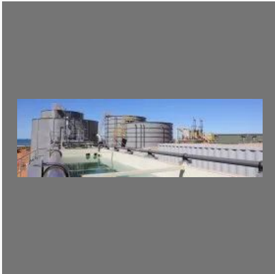
Residential Water Management Service
