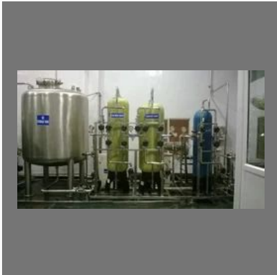
Demineralised Water Plant
