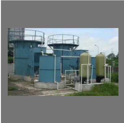
Sewage Water Treatment Plant
