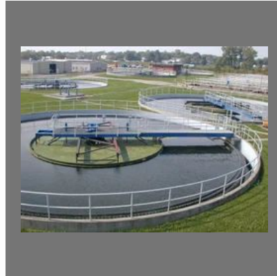
Commercial Water Treatment Plant
