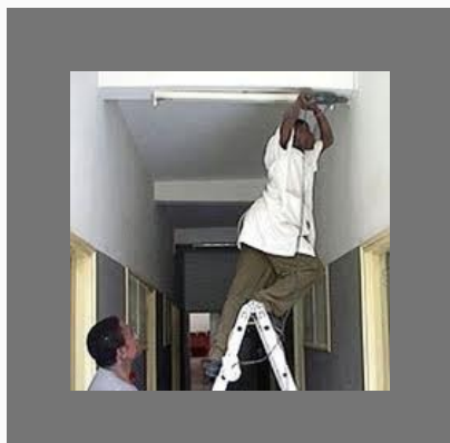
Internal & External Wiring for Offices
