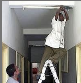
Internal & External Wiring for Offices
