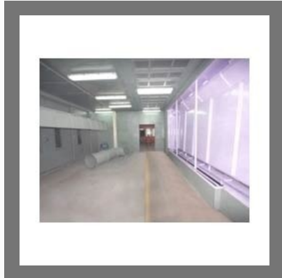
Water Curtain Type Paint Spray Booth
