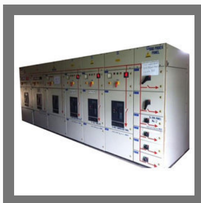
Three Phase Power Panel
