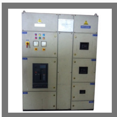
MCC Starter Panel
