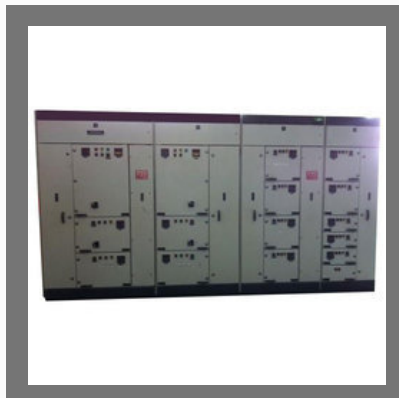
LT Distribution Panel
