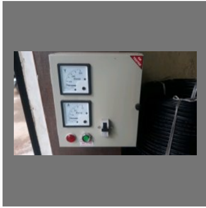
Electric Control Board
