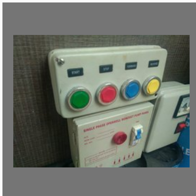
Control Panel Board
