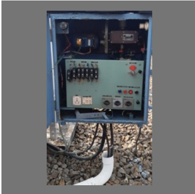
Isolator Drive Boxes, MOM Boxes
