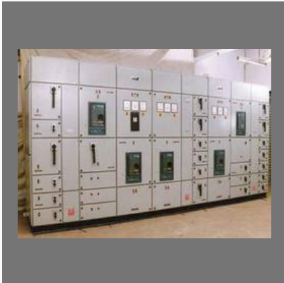
PCC Control Panels
