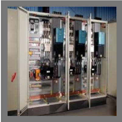
MCC Control Panels
