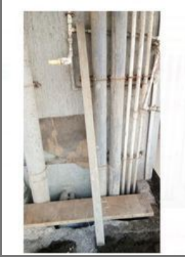
Pipe Fitting Service
