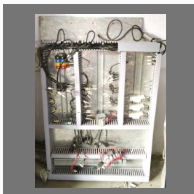
Construction Machinery Control Panels
