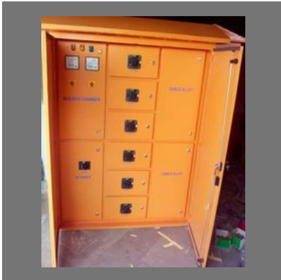
Control Panel Board
