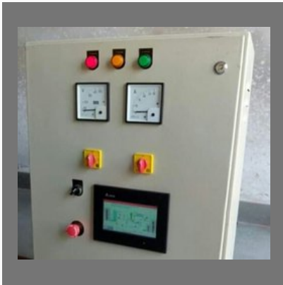
Electric Control Panel
