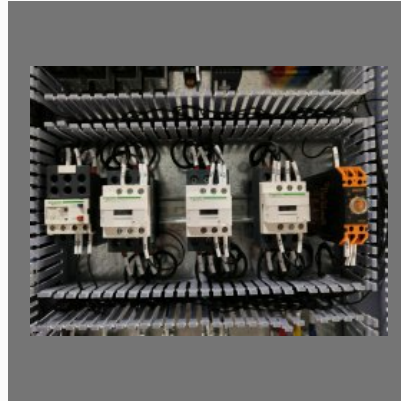
Electric Control Panel
