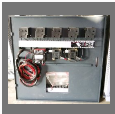
Industrial Control Panel
