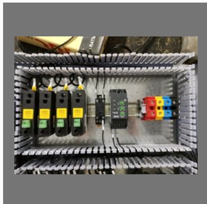
Electrical Control Panel
