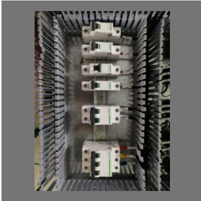
Electric Control Panel
