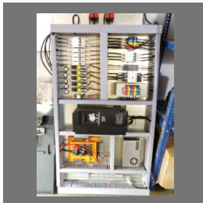
Electric Control Panel
