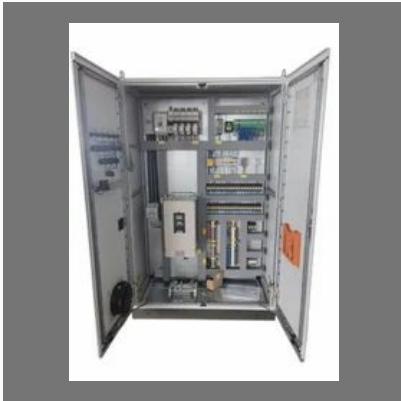
415V Automation PLC Control Panel
