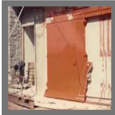
M.s. Shielding Sliding Doors
