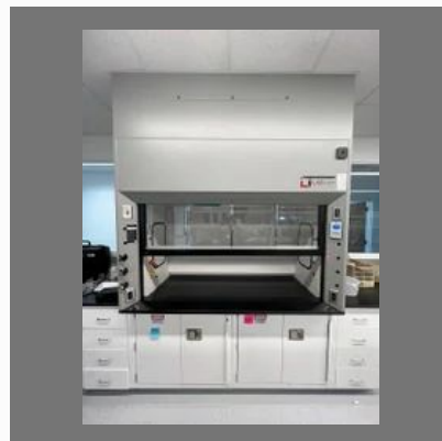
Laboratory Fume Hood
