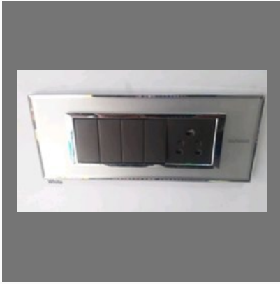
Designer Switch Board
