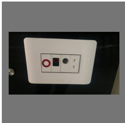
TV Cable Switches
